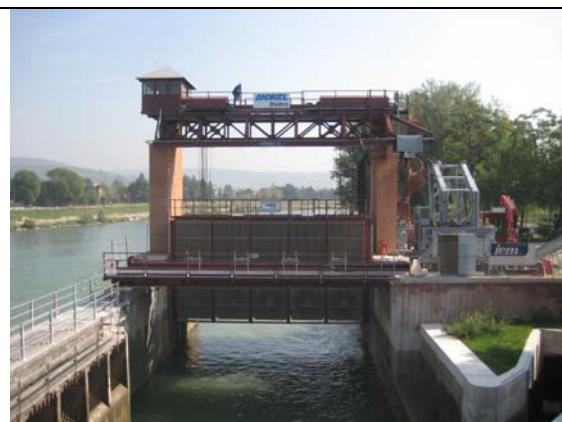
Picture 4: The Chievo dam HYDROMATRIX® plant seen from the upstream side. The Module is lifted out of the lock's water passage. On the right side of the lock wall, the upstream entrance of the newly constructed fish ladder can be seen.
