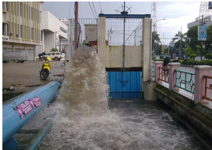
Figure 13. Pumping system for Bendung Sub-cathment
