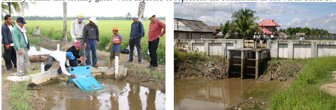
Figure 3. Example of movable flap gate in a tertiary canal and a flap gate in a secondary canal
