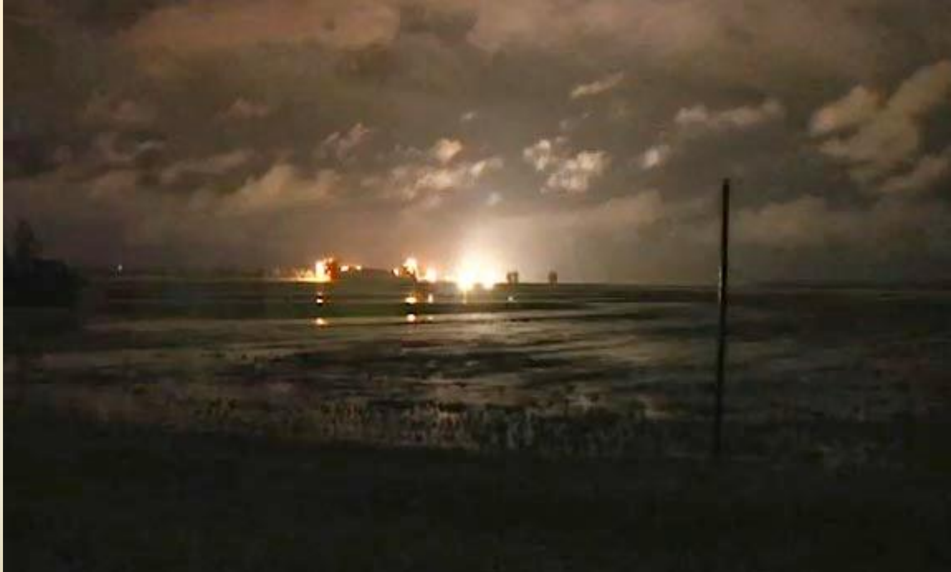
Army Corps of Engineers 's demolition of the Birds Point levee on the Mississippi River on May 2, 2011.
